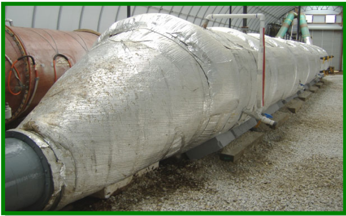
Avatar's experimental modular plug-flow digester
